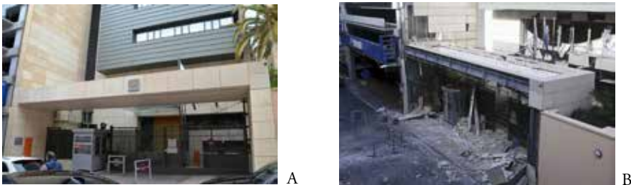
Image 2. Embassy of the Republic of Cyprus in Athens: entrance area, state before the explosion (A), state after the bomb explosion (B).
